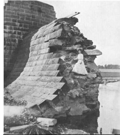
This shows the effects of the 1905 dam break. The area had received over 11 inches of rain in 16 hours. A Pictorial History of Bridgeport by David Palmquist, 1981
